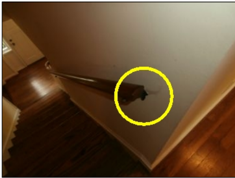
open ended handrail
