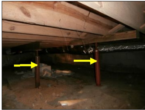
auxiliary floor posts
