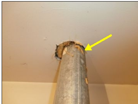
deficient clearance from combustible material
