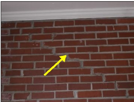
crack at side B of carport
