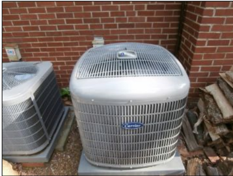
air condensing unit
