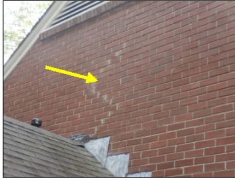
sealed crack at side B
