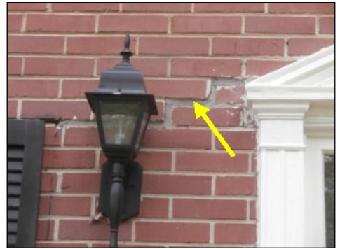
previously sealed crack at side A
