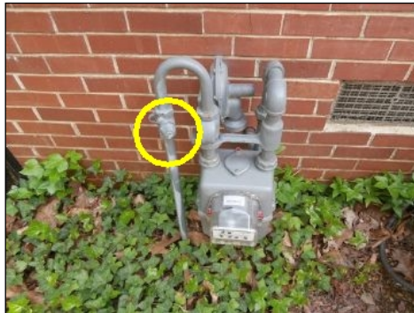
main gas valve
