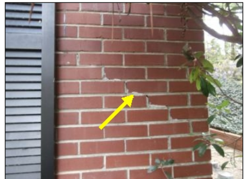
previously sealed crack at side A
