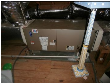
general image of heat pump
