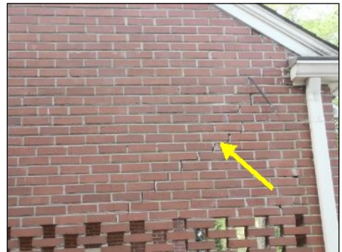
step crack at side B of carport
