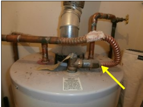
improper discharge tube installation
