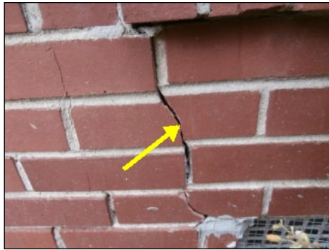
open crack at side A
