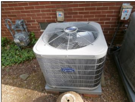
air condensing unit
