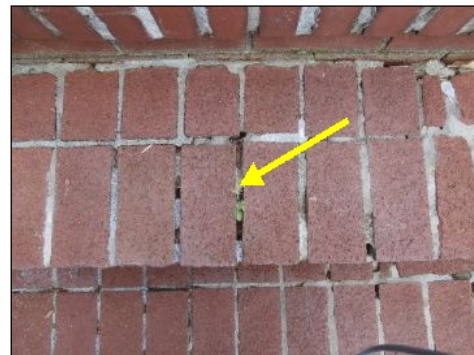
missing mortar example
