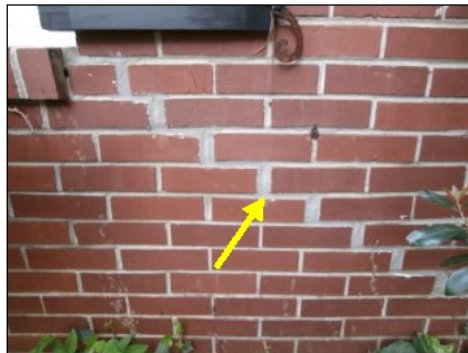
previously sealed crack at side A
