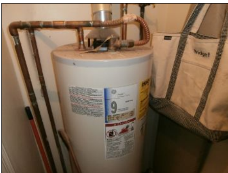
general image of water heater
